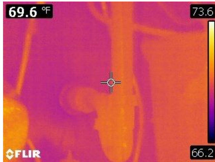
No clogs detected in sink trap
