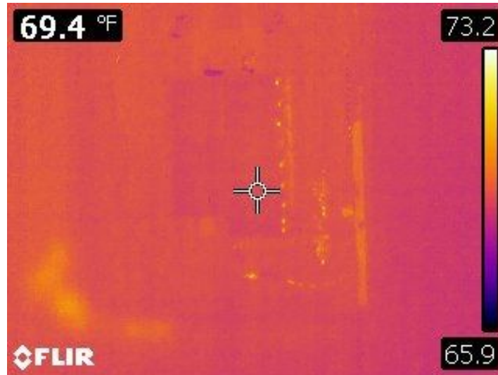
Sub-panel in living room
