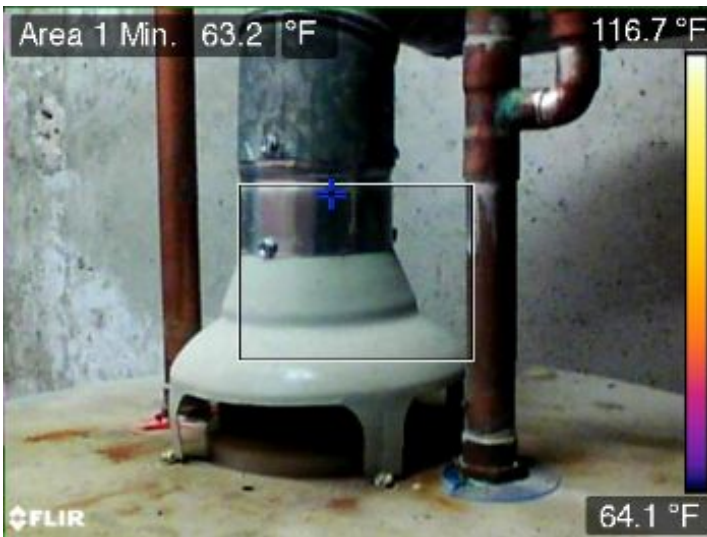
Hot water tank
